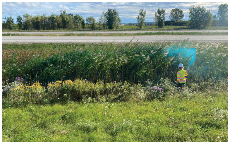
Phragmites treatment within roadside ditch
